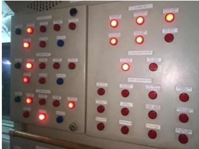
Figure 3. Alarm signalling panel [2]
