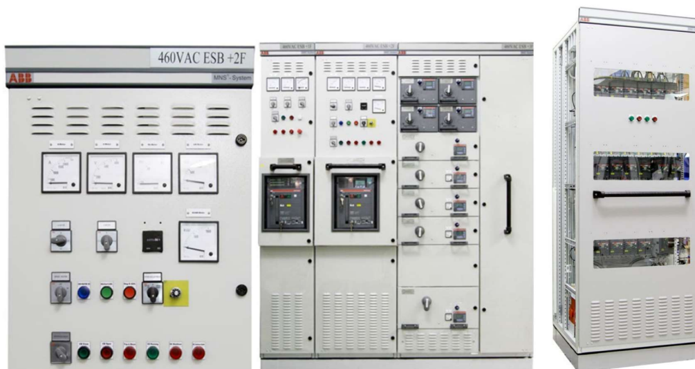
Figure 4. Synchronizing and distribution cubicle of MNS 3.0
